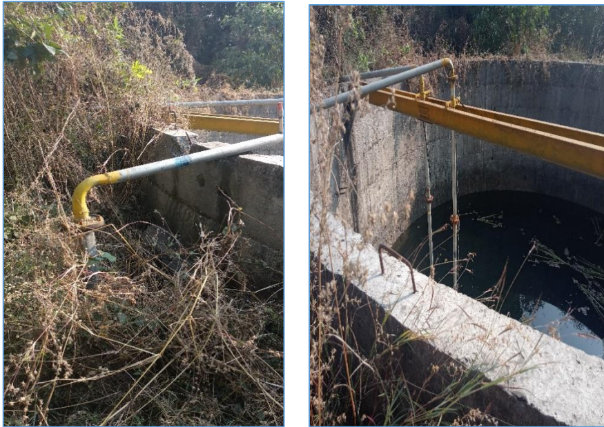
Figure 8.6.6B: Submersible pump and pipe connected to pump and proper support structure
