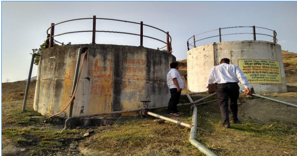
Fig8.6.6D: Two Ground Storage Reservoirs
